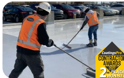
Chamberlin Roofing & Waterproofing won 2 nd place for the “OU Research Parking Garage” project.
